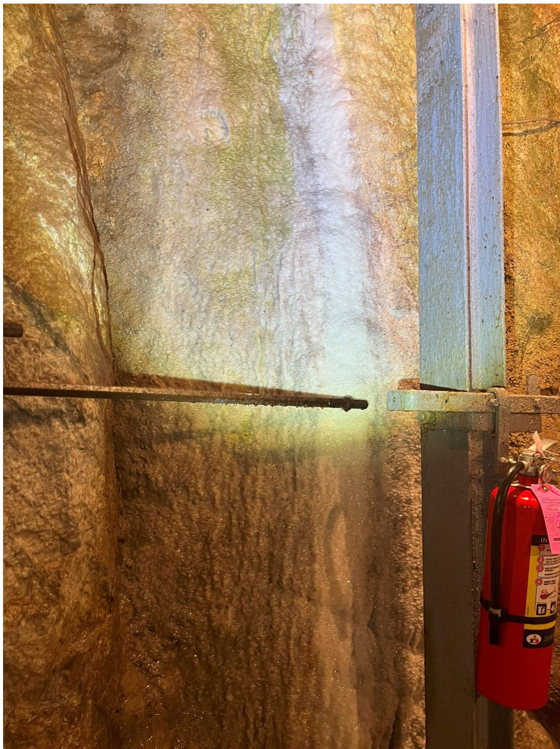
Figure 5. Behind the galvanized I-beam the flowstone varies in color. The green color is due to algae, which can grow here because the tour lights provide enough energy for photosynthesis to occur. Note the white vertical stripe in the photo; no algae grow in this area because it lies in the shadow of the I-beam.
