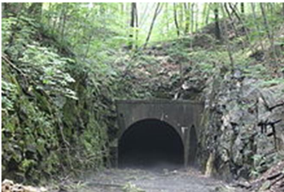
Figure 3. The eastern portal of Oxford Tunnel on the Old Road in August 2011.
