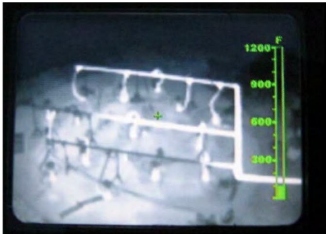
Figure 16: A) Infrared photograph of Thermal Conductive Heating well array. Photo at night showing hot recovery and cold recovery pipe sections.
