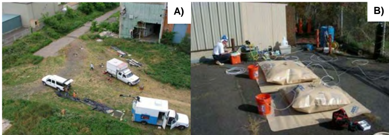
Figure 12: A) Photo of Shapiro/USGS P&T, MNA, and EB research Site, B) Photo of bags filled with EOS to be injected into research well 36BR
