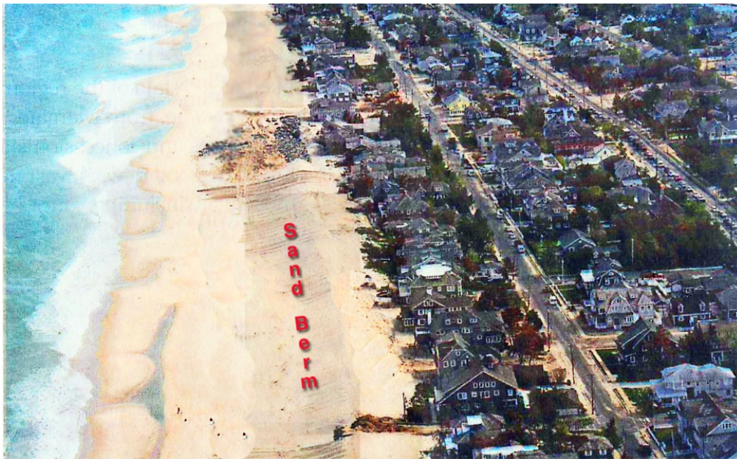
Figure 12. Construction of a sand berm along the northern New Jersey Coast after Hurricane Sandy (2012).
