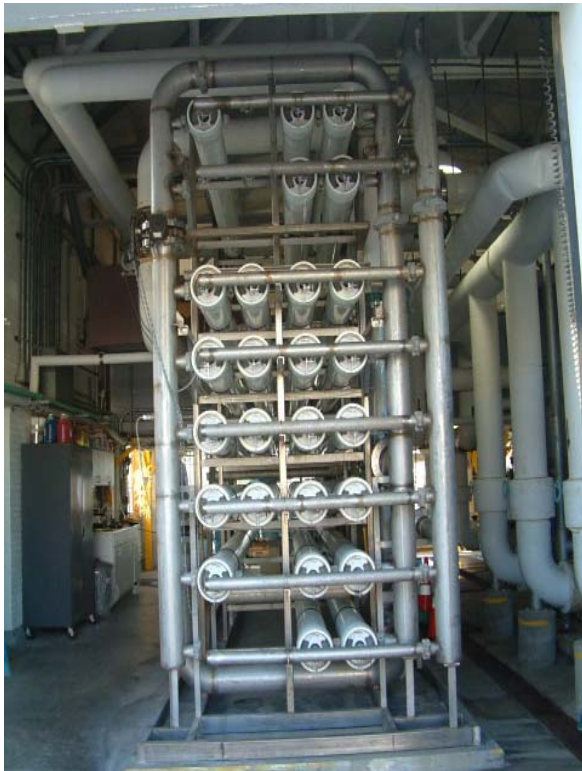
Figure 13. Desalination units of the Cape May City desalination system (photo from Carl Behrens Cape May City Water Department )
